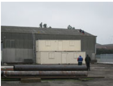
The two men working in unsafe conditions on the roof
