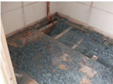
Loose fill blue asbestos insulation in the area where Mr Arnold had been working
