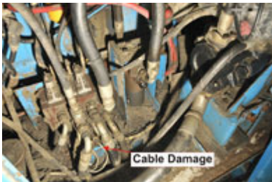
Location of damage to cable
