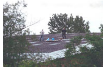
The roofers spotted by a passing HSE inspector
