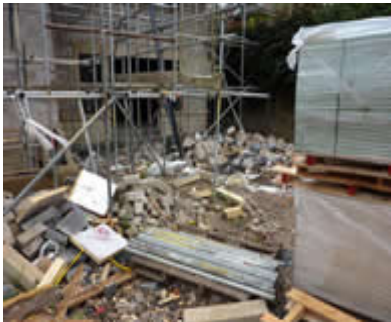
Inspectors found large amounts of rubble around the site making access dangerous
