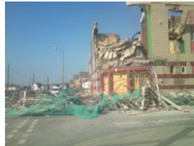
The collapsed cinema in Thornton Cleveleys
