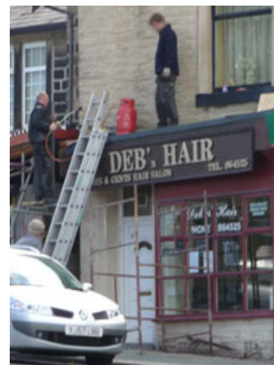
Ross Singleton (left) and another worker carrying out work on the roof of a hairdressers' in Colne
