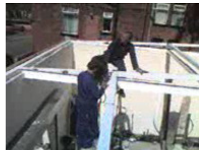
Video image taken from John McCleary's mobile phone showing the unsafe work
