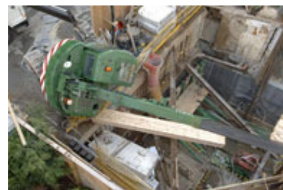
The overturned mini-crawler crane which crushed Mr Page
