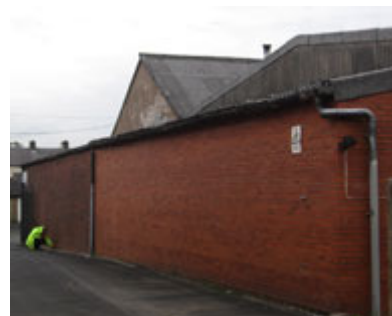
The roof from which the worker fell
