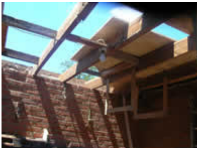
The gap in the roof through which Mr Waughman fell
